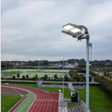
Example image of column mounted sport lighting
